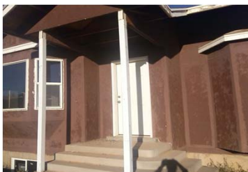
Needs stucco finish
