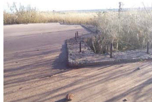
Poor quality concrete work
