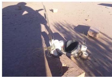
Brittle and damaged plumbing
