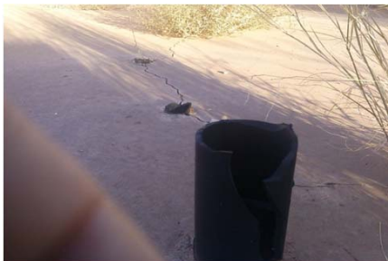
Brittle and damaged plumbing
