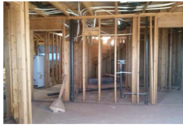
Additional framing needed
