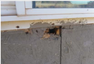
Weather damaged exterior
