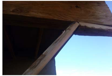
Additional framing needed
