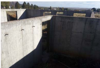
No Plumbing or Electrical
