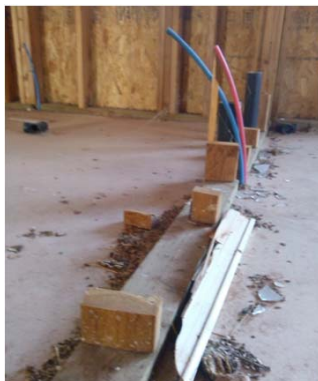
Additional framing needed
