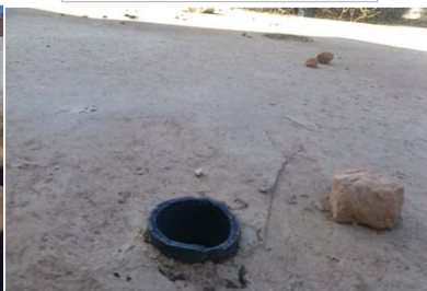
Brittle and damaged plumbing
