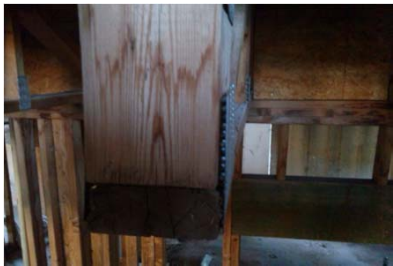
Weather damaged trusses
